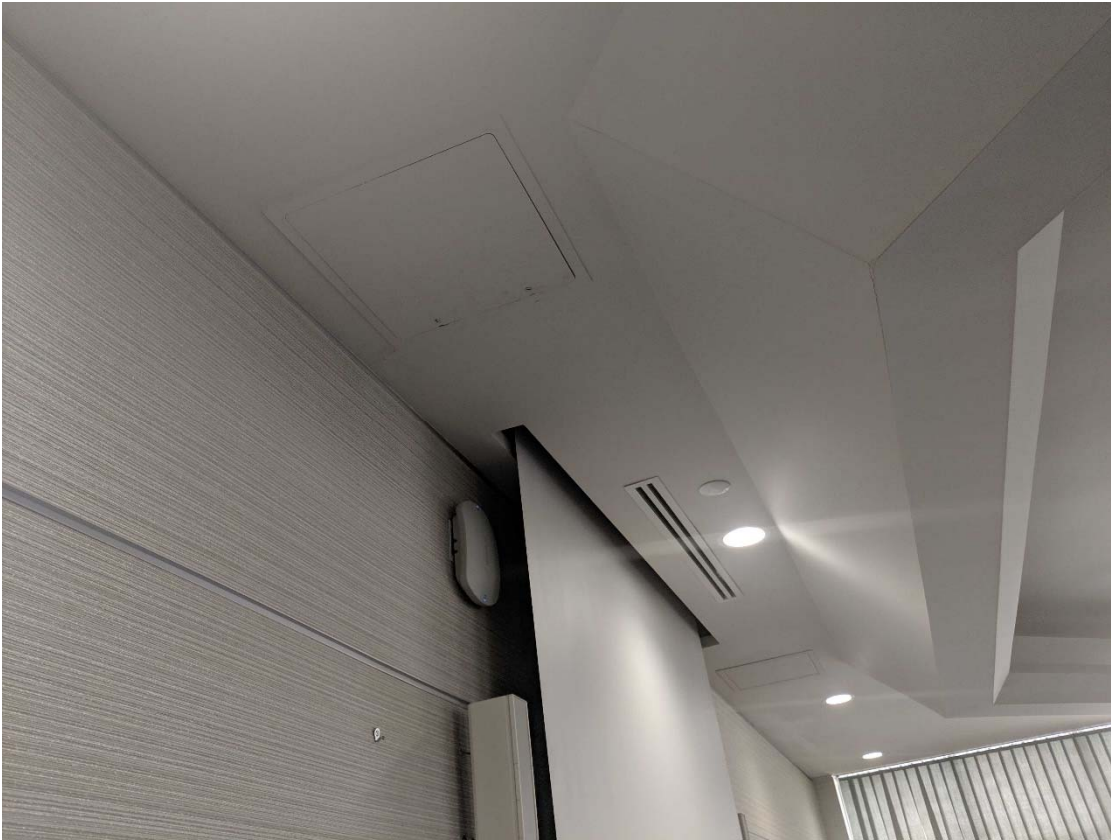
Figure 8 - Projector screen and access panels
